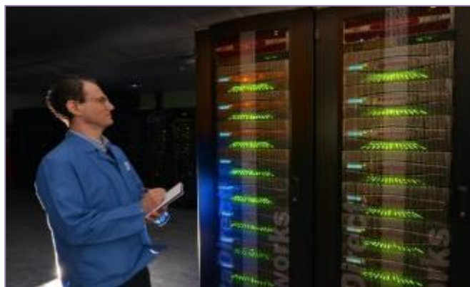
WCDI Computer Racks
